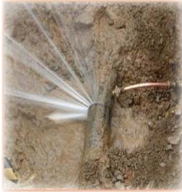
A Leaking Water Main
